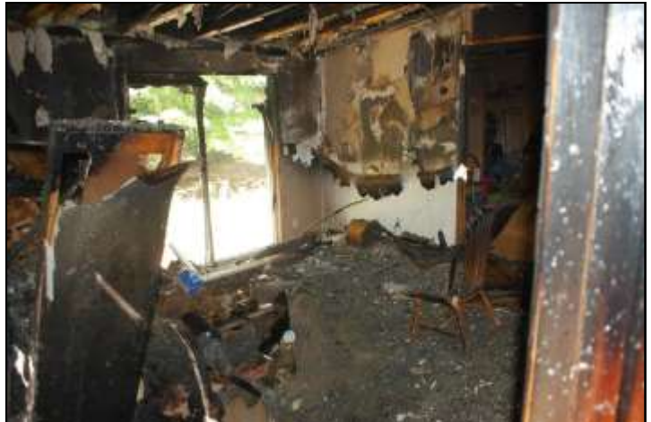
Dining room with floor collapse.
