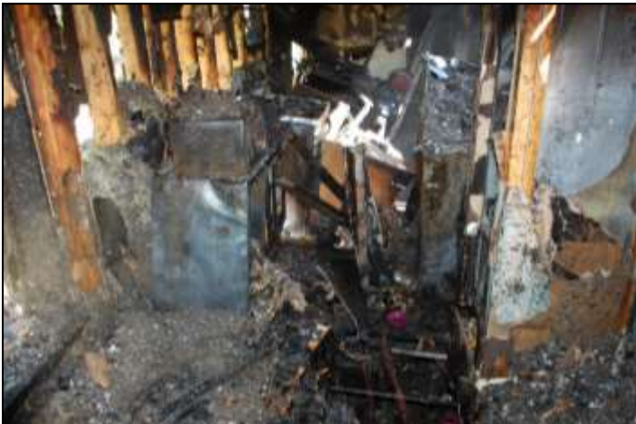
Kitchen with floor collapse.
