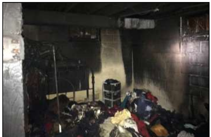
Smoke damage from a basement fire.
